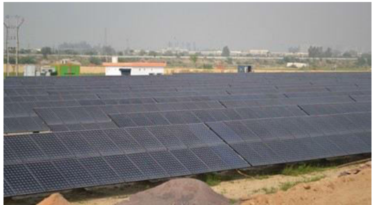
1MW Ground Mounted Solar Plant Kasna, Gr. Noida
