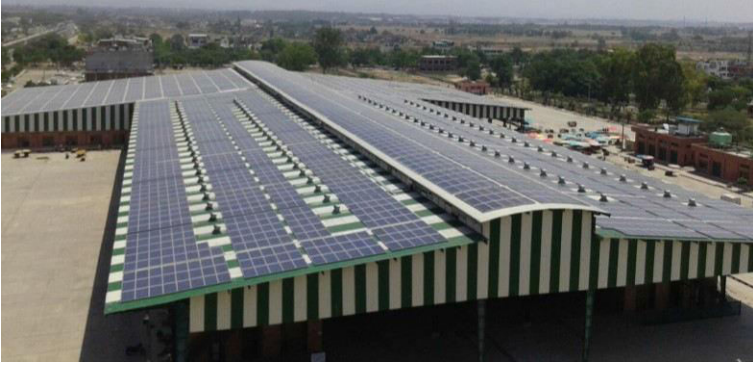
2.56MW Single Rooftop Solar Plant-SAS Nagar, Mohali, Punjab
